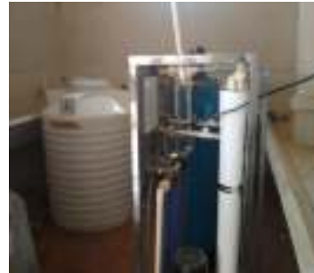
RO Plants installed in TW Institutions
